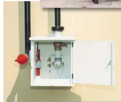
Ground Level Spill Box
